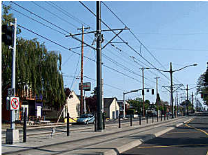
Ugly Overhead Wires
